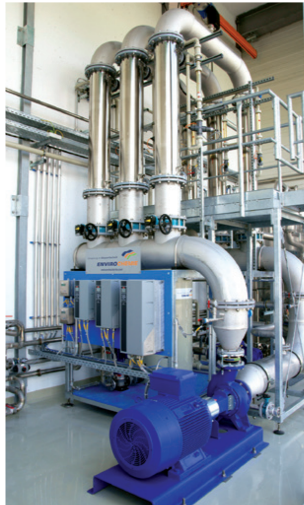
Recovery of solvents (© EnviroChemie GmbH)
